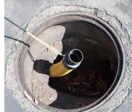
Tiger tail used on a manhole
